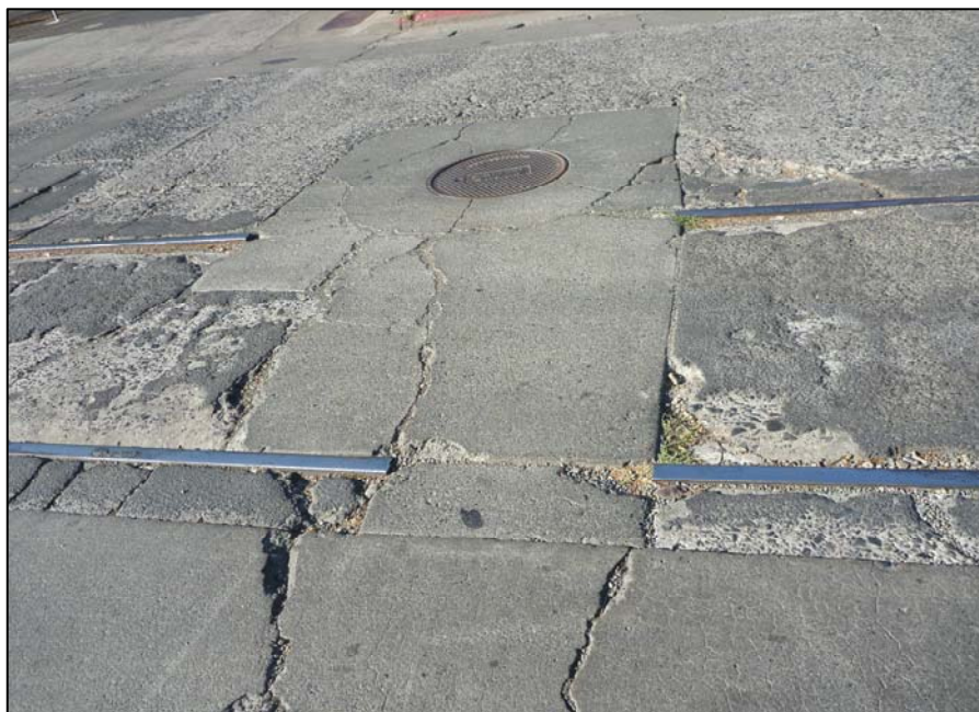
Figure 14: Sections missing from each rail.
