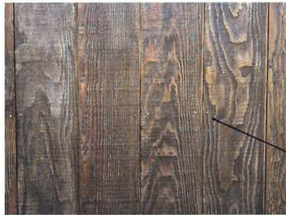
STAINED VERTICAL WOOD SIDING
