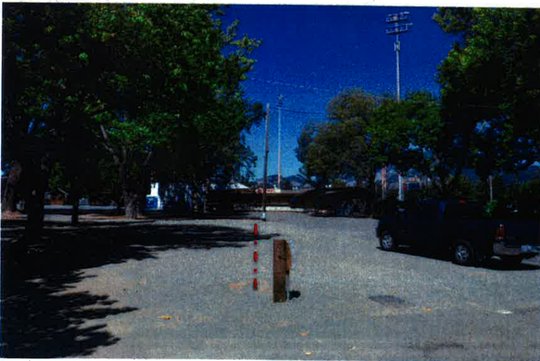
Post is AT&T fiber point of connection. Underground utility run is to pole in background and then to equipment shelter to trees on right.
