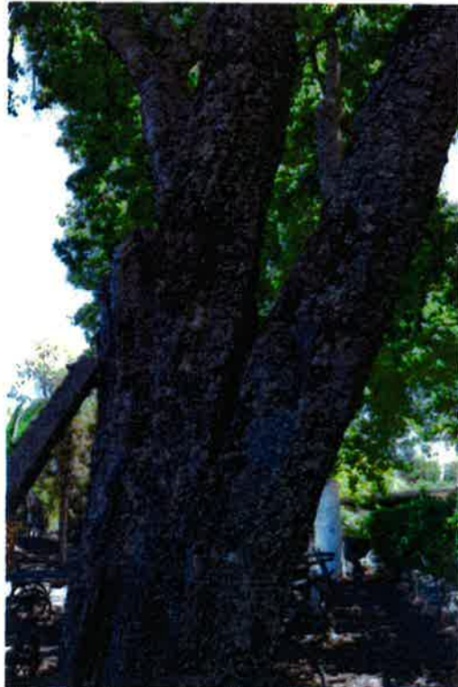
Fissure at trunk union of tree #2. Trunk is at risk of failure.
