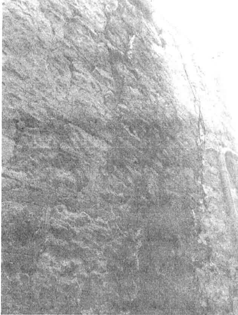
Photo3 – West wall crack
