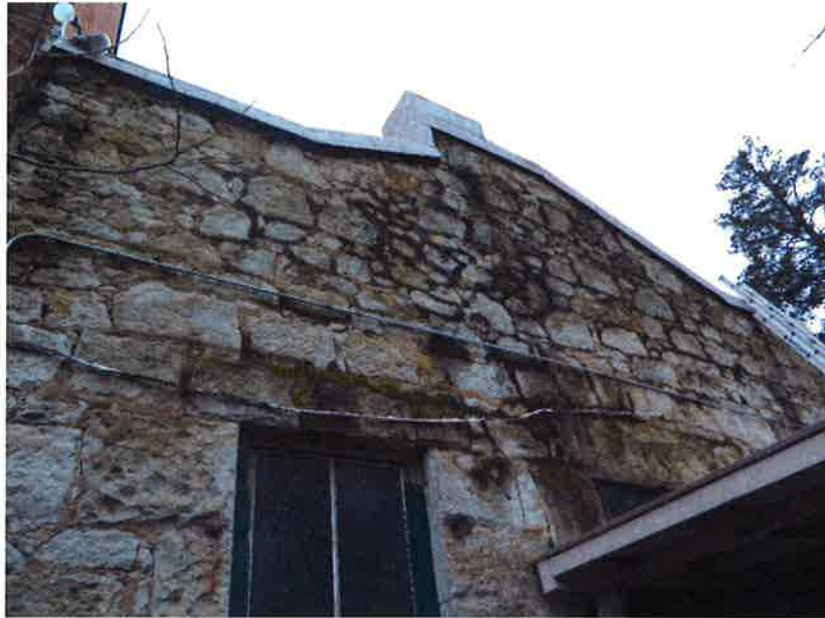
Figure 16. Irregular shaped roof cornice on the west elevation, showing repointing and staining.
