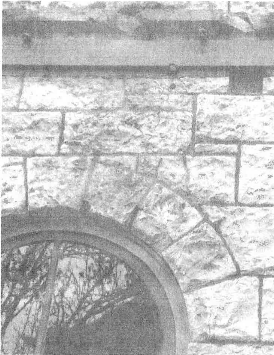
Photo 2 – Façade east window header
