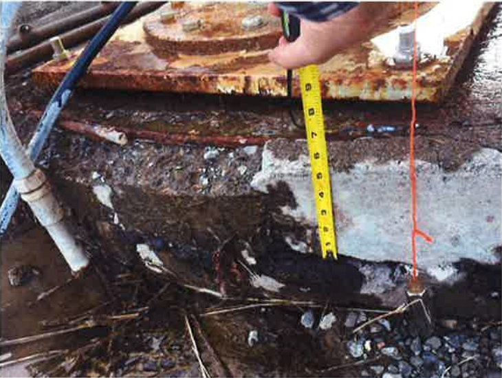
Photo 2 – Failing Flat Top Lid
