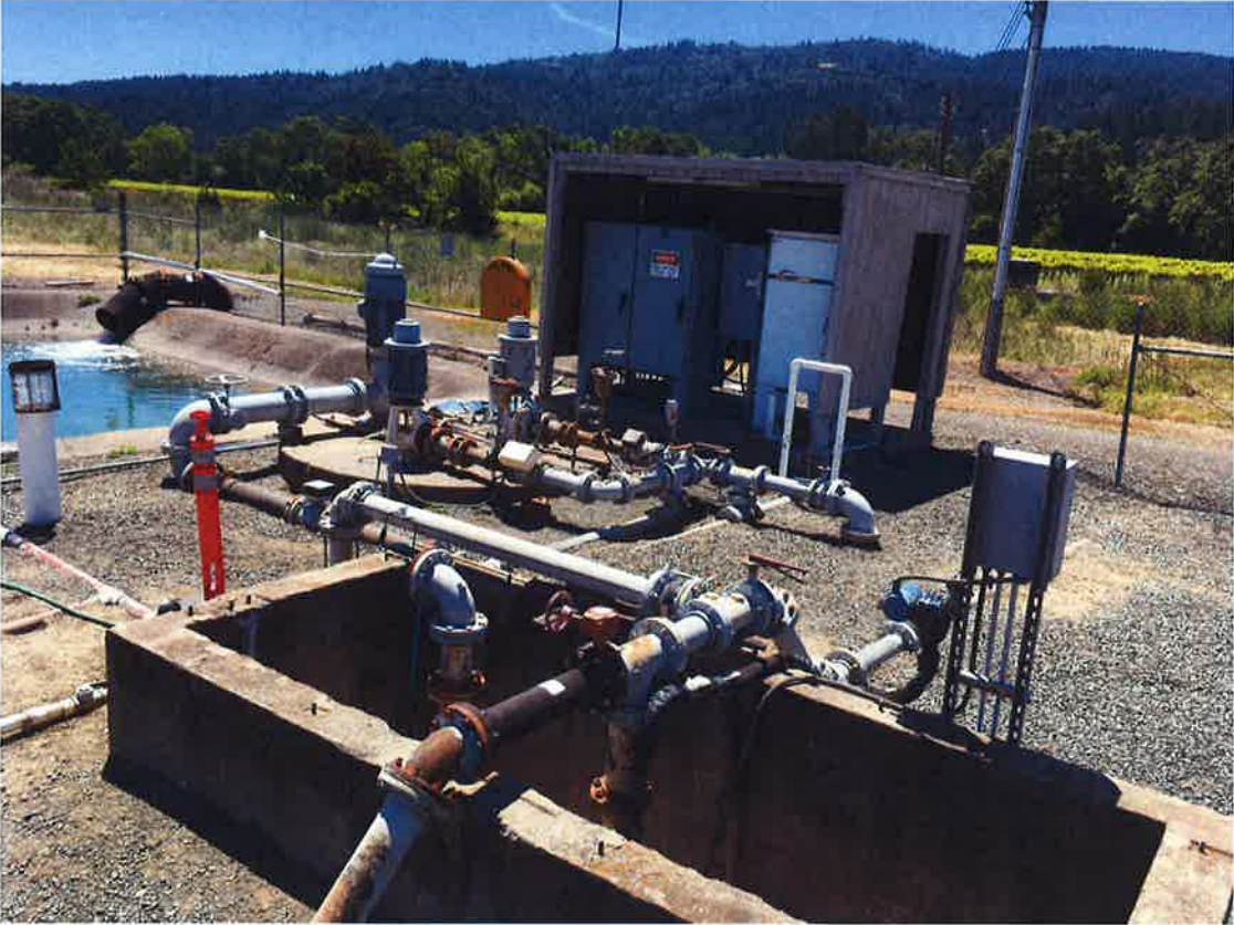
Photo 1 – Existing Irrigation Pump Station
