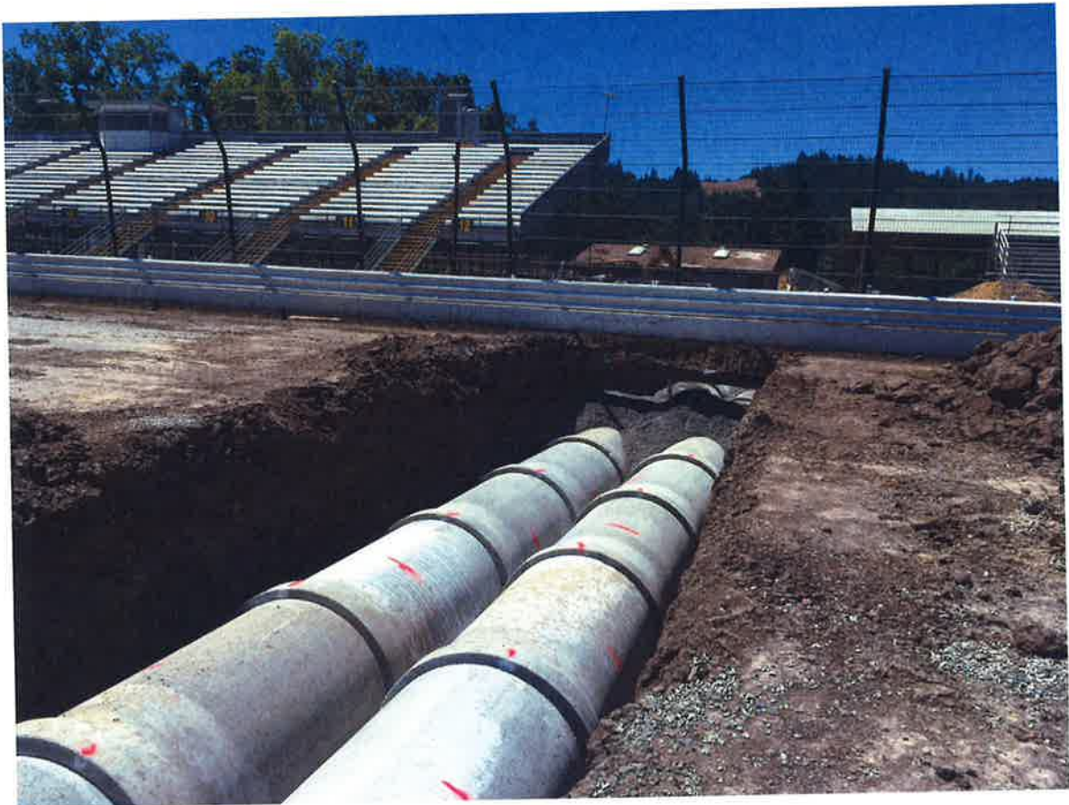
GRANT STREET STORM DRAINAGE UNDER RACE TRACK
