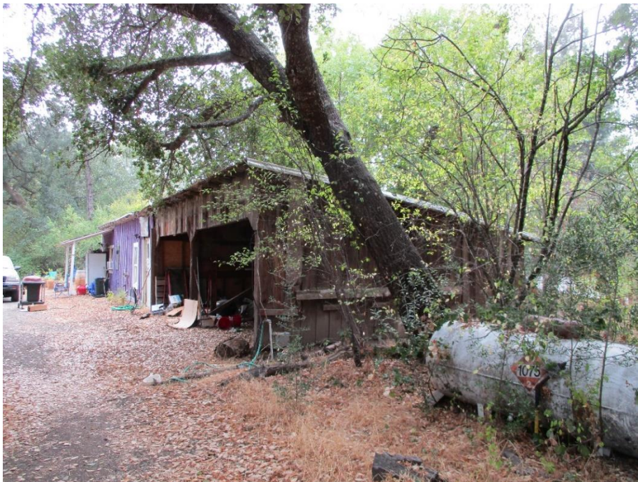
Figure 4. Photograph showing the east elevation, and horizontal boards along the wall, facing west.
