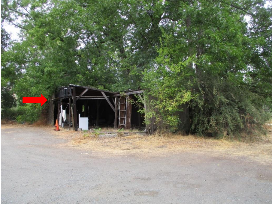
Figure 6. Photograph showing the northwest corner of the ca. 1950 barn, with fire damage along the shed roof (red arrow), facing east.
