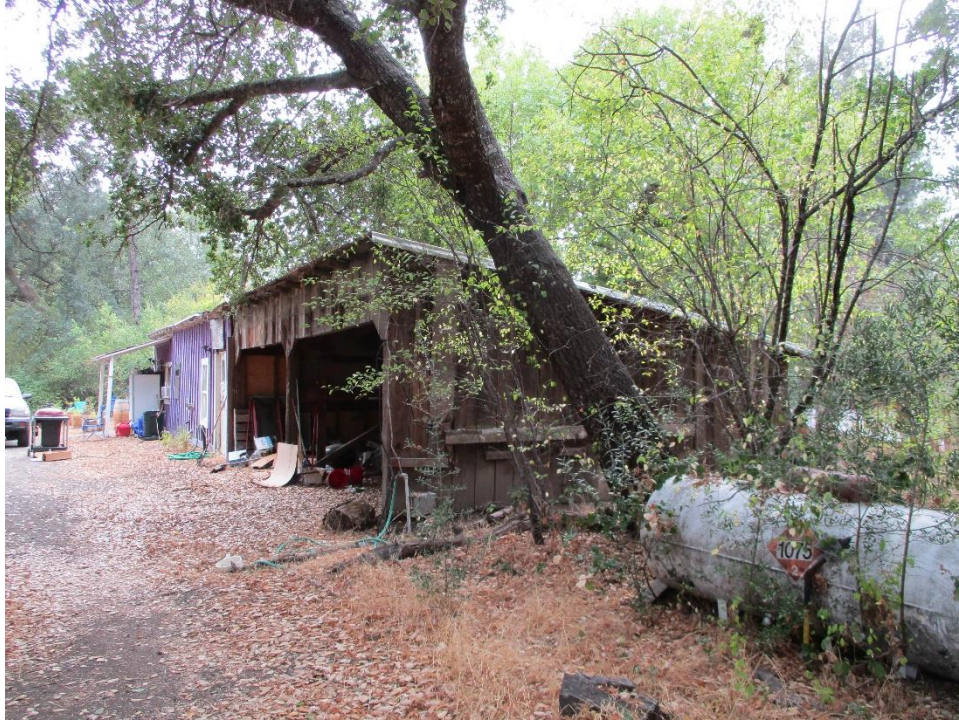
Figure 18. Photograph showing the east elevation, and horizontal boards along the wall, facing west.
