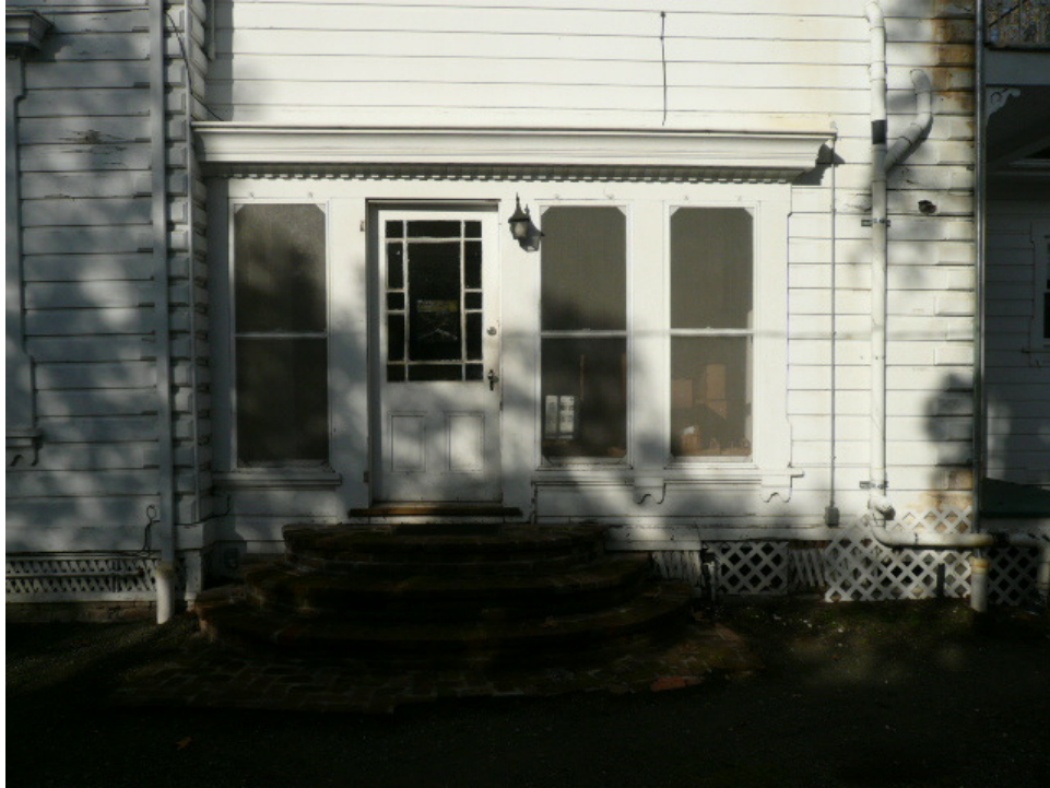
View of east elevation from outside family room. Window on left to be removed, and door, two windows to be replaced with conforming style (one over one) wood windows
