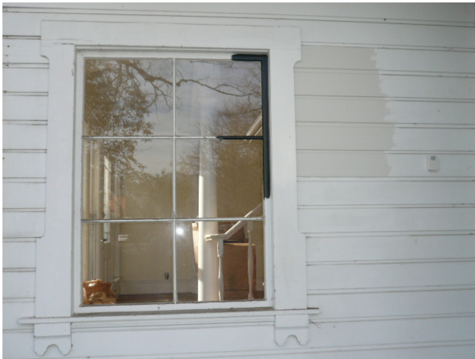
Window at north elevation to be replaced with conforming (one over one) wood window. Paint samples visible on window trim and siding to right of window
